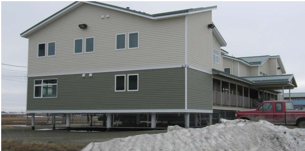
Figure 29. People's Learning Center ("Yuut Elitnaurviat" in Yupik Eskimo). This learning center in Bethel has an open crawl space.
