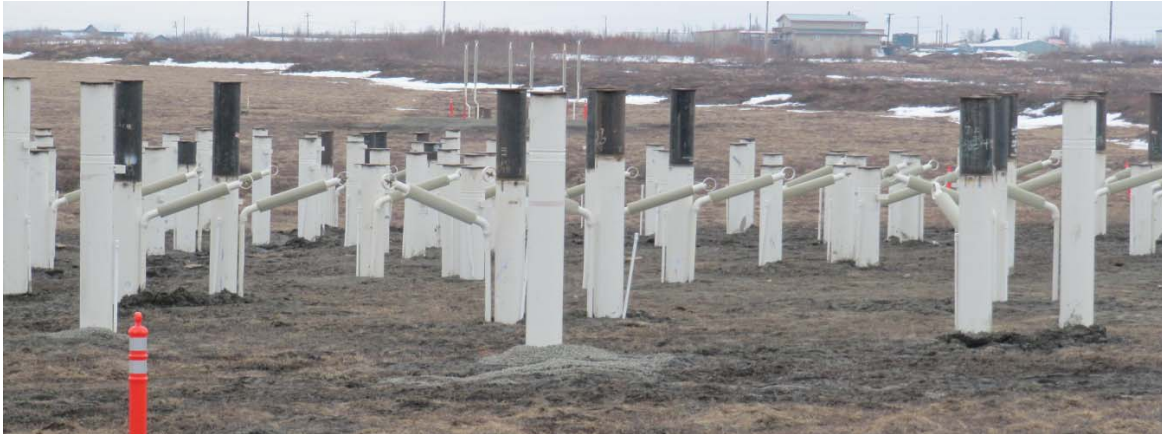
Figure 32. Thermopile installation normally occurs well before building construction. The thermopile radiator sections (tilted out from the vertical piles) are clearly visible.
