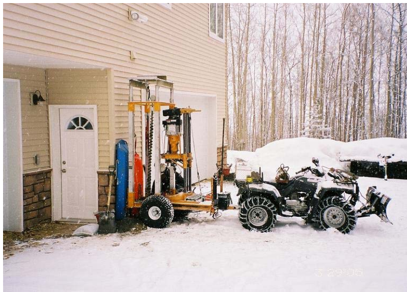
Figure 15. Using a smaller drill rig permitted boring thermistor holes closer to the building. During the drilling operation, we used screens to protect the building.
