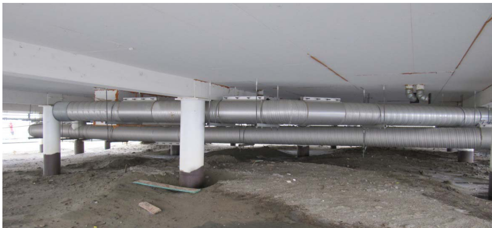
Figure 30. Utilities protected from freezing by enclosure within insulated arctic pipe.
